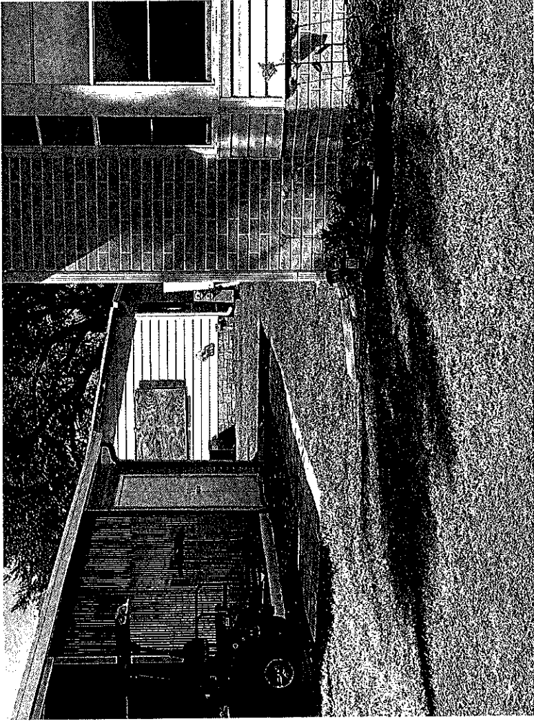
Photo: 439 Royal Tern (rear). Post-V.C. re-inspection. Plywood not painted to match house.
