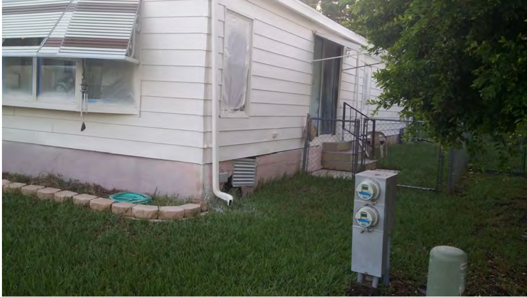
Photo: 446 Marlin (right side). Skirting damage.
