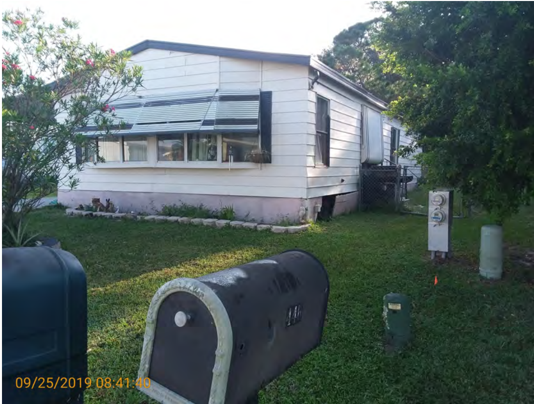
Photo: 446 Marlin. Post-V.C. re-inspection. Skirting damage.
