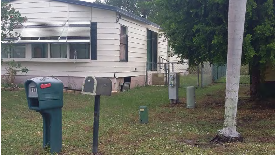
Photo: 446 Marlin. Post-V.C. re-inspection. Skirting damage.
