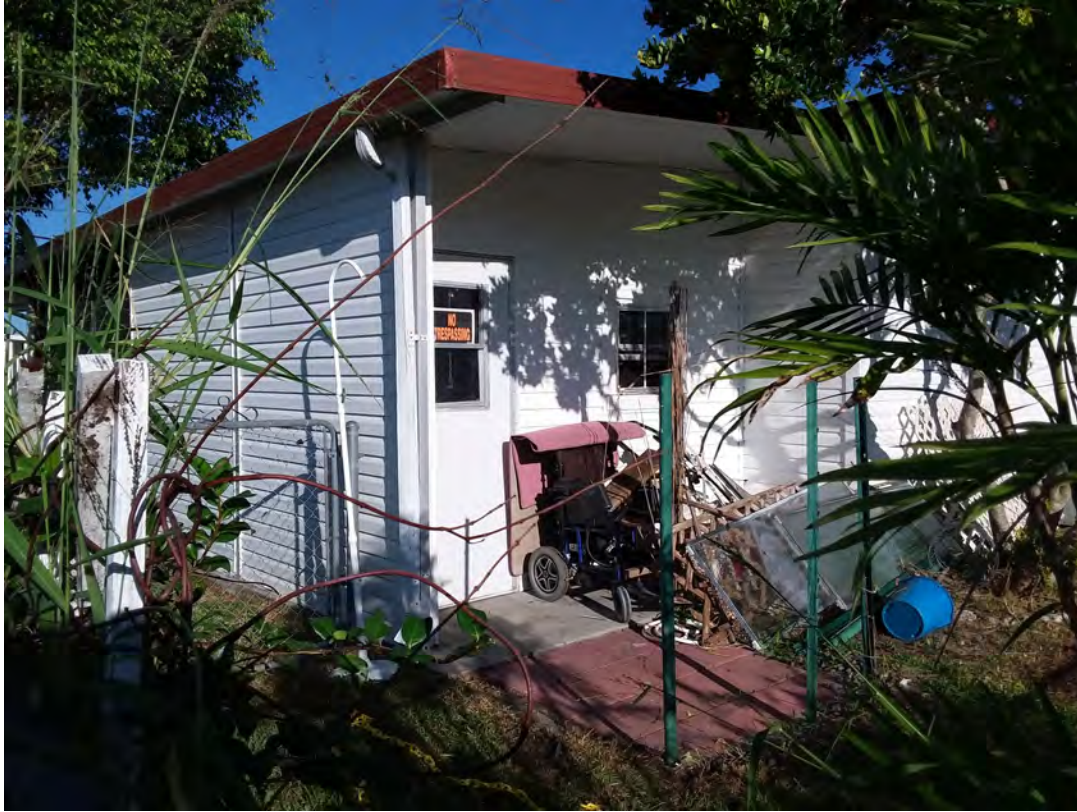
Photo: 915 Wren. Unapproved items - Debris
