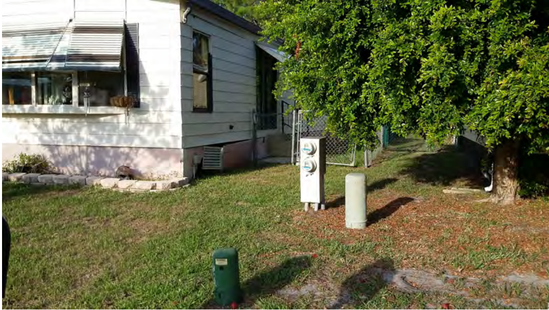
Photo: 446 Marlin. Post VC re-inspection. Skirting damage.
