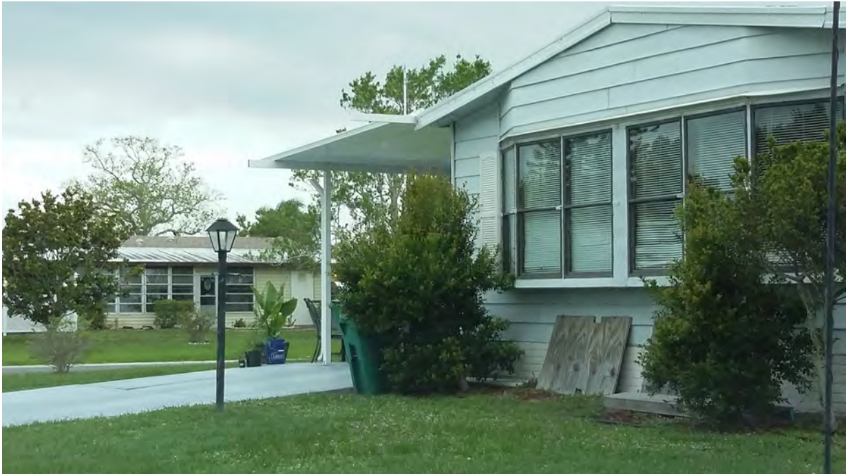
832 Oleander. Carport roof damage Mary Barry May 15, 2019
