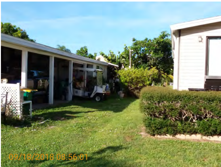
709 Wedelia Roof, fascia, gutter-IRMA Terri Curles Sep 18, 2018
