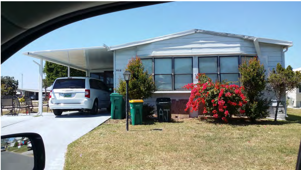
832 Oleander. Carport replaced, still has fascia damage. Peter Essig Mar 18, 2018
