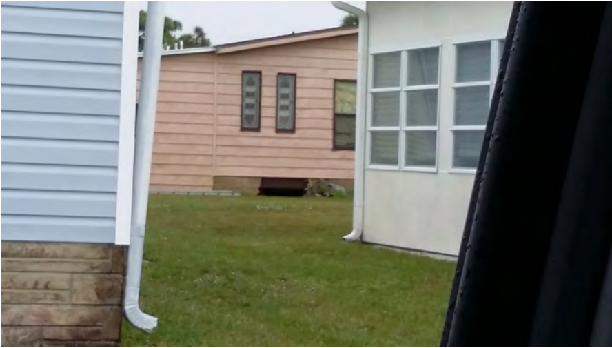
516 Egret (rear). Skirting damage. Peter Essig Mar 19, 2019
