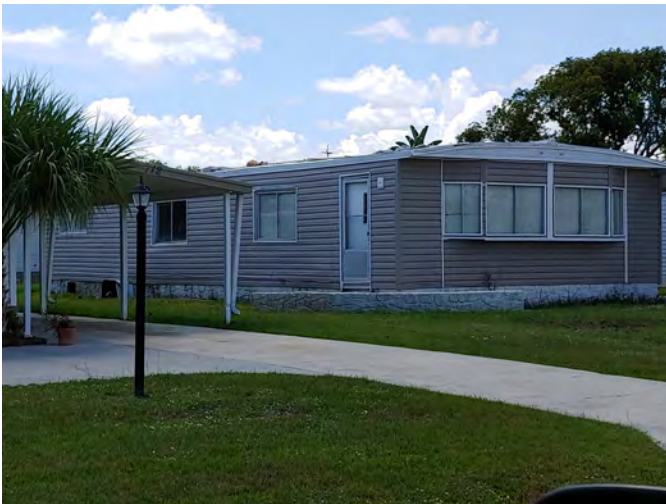
710 Lark roof and siding damage Stephane Fecteau Jun 03, 2019
