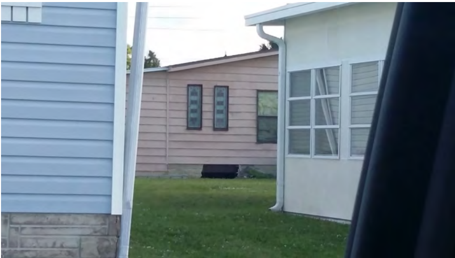
516 Egret. Skirting damage. Peter Essig Apr 17, 2019
