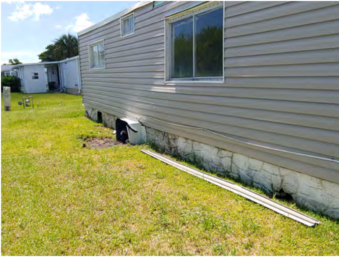
710 skirting damage Stephane Fecteau Jun 03, 2019
