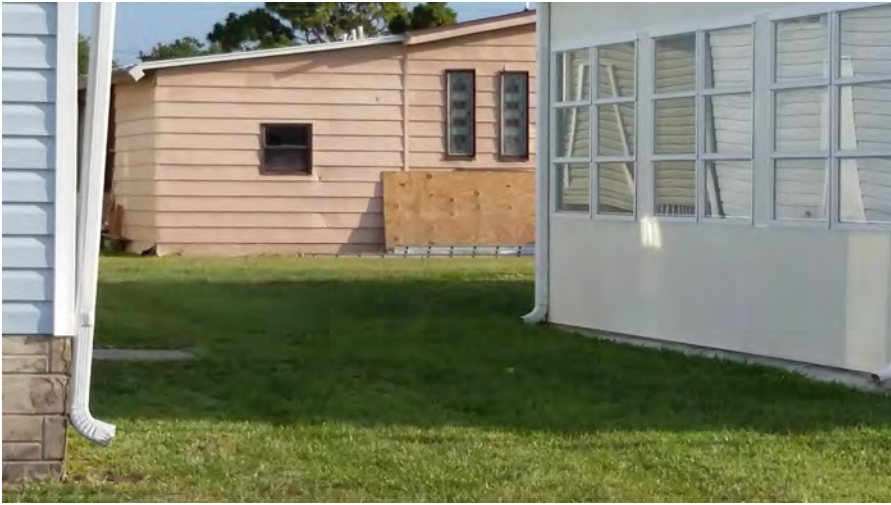
516 Egret (rear). Siding damage (utility room/shed) Peter Essig May 28, 2019
