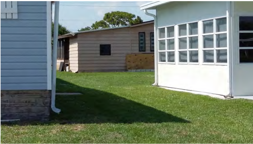
516 Egret (rear). Pre-VC inspection. Skirting damage (plywood used to hide damage) Peter Essig May 07, 2019
