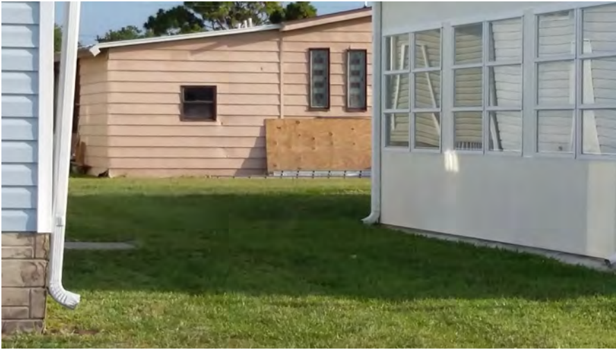
516 Egret (rear). Post VC inspection. Skirting damage (hidden by wood) Peter Essig May 28, 2019
