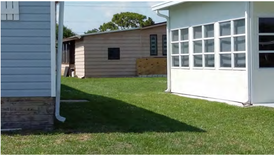
516 Egret (rear). Pre-VC inspection. Siding damage (bottom of utility shed) Peter Essig May 07, 2019
