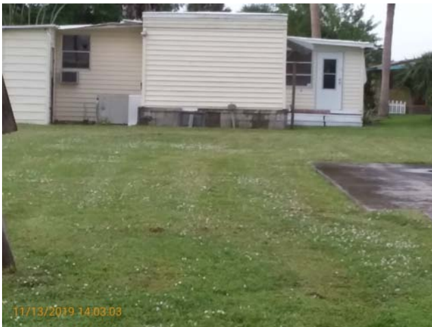
891 Pecan. Concrete block used to hold up vent cover Nov 13, 2019
