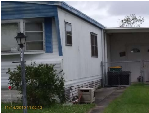
861 Cashew. Siding damage, window damage Nov 14, 2019
