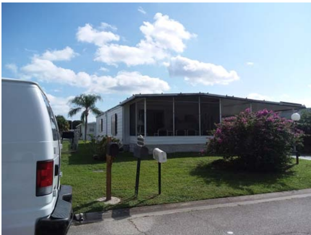
919 Wren. Exterior maintenance Fascia damage- needs paint.
