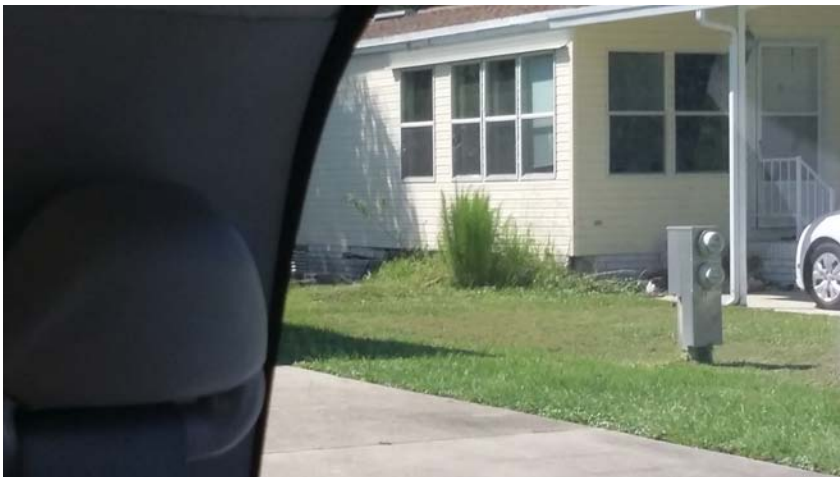
1042 Sebastian. Skirting damage. Sep 17, 2019
