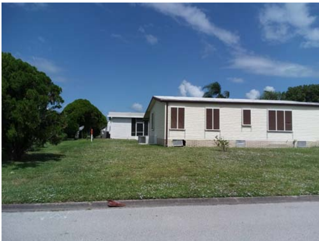
701 Bougainvillea. Skirting needs to be replaced / repaired. Oct 01, 2019
